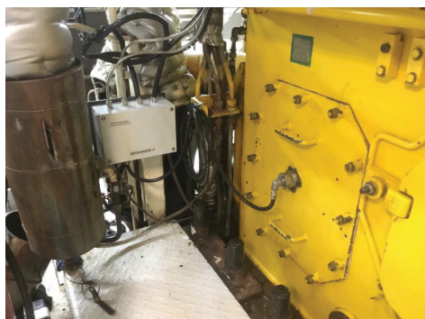
Junction Box & Sensor Installation am Motor
