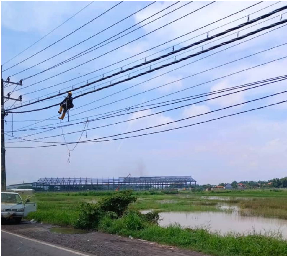
A new factory being constructed behind Spiderman fixing the cable. Gresik, East Java.
